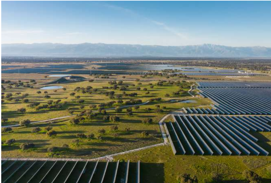
Location: Talayuela Solar Plant, Spain
